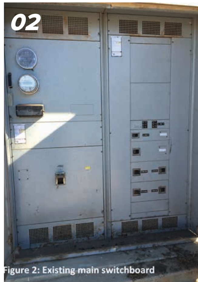
Figure 1: Existing main switchboard
