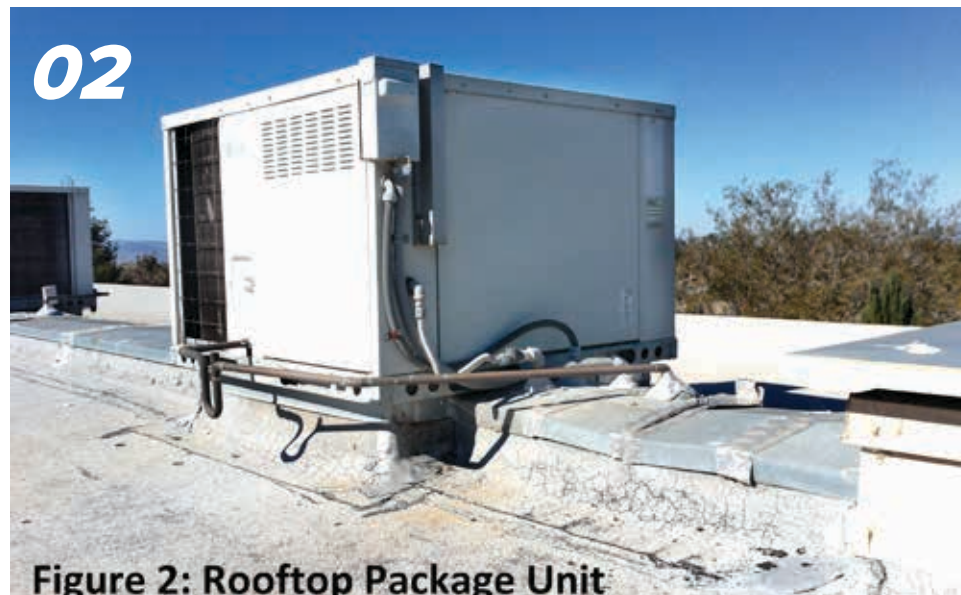
Figure 1: Rooftop Package Units
